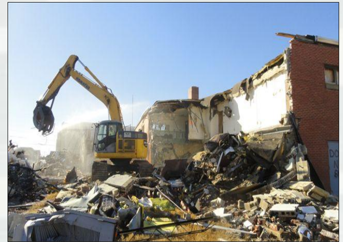
An excavator demolishes the former U.S. Army Reserve Center in Tuscaloosa, Ala. The center and surrounding buildings were hit by a tornado.
