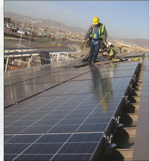
The Brigade Combat Team Dining Facility at Fort Bliss, Texas, is powered by solar panels.
