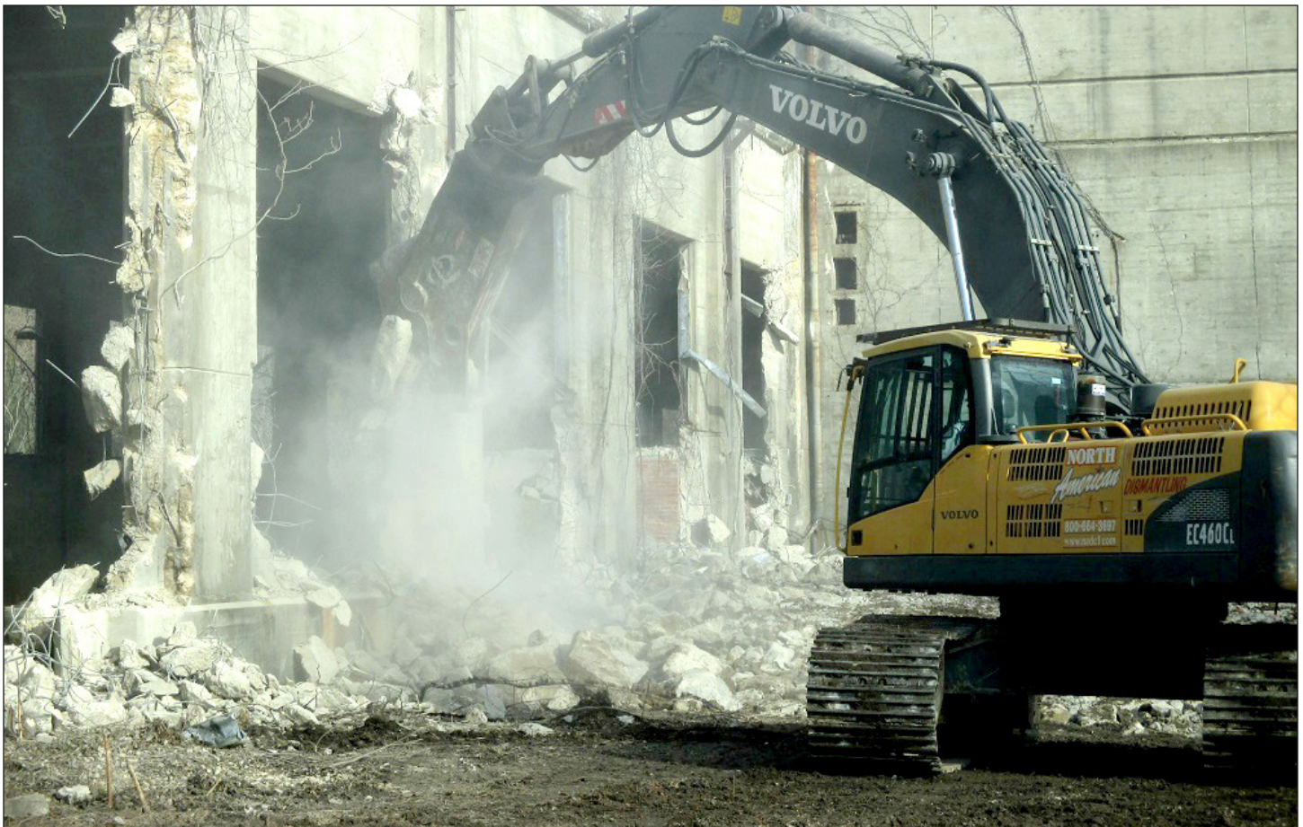
By the mid-1980s, the Huntsville Division's evolving mission included removing excess facilities from installations, such as the heat plant shown here at U.S. Army Reserve Weldon Spring Training Area, St. Charles, Missouri. (Photo by North American Dismantling Corp.)
