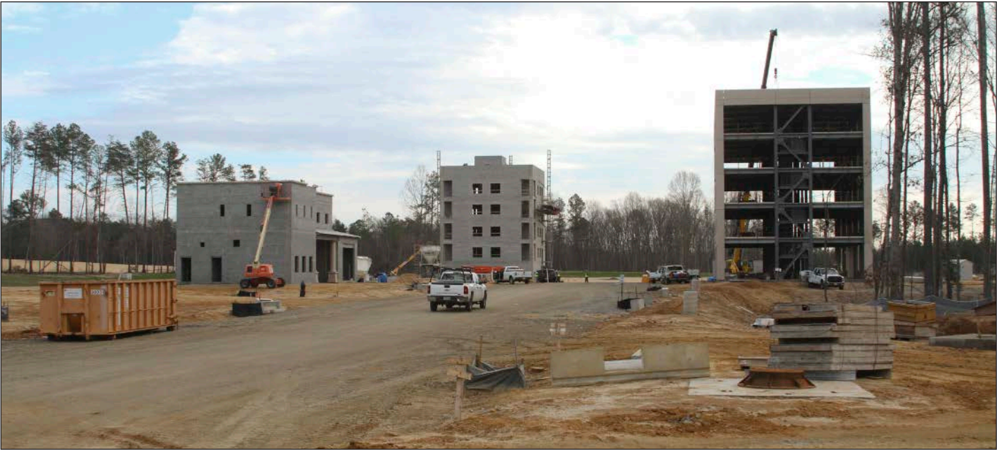
The construction of military operations in urban terrain, or MOUT compounds at Fort Irwin, California, and Fort A.P. Hill, Virginia, shown above, were overseen by the Huntsville Center's Range and Training Land Program Mandatory Center of Expertise.
