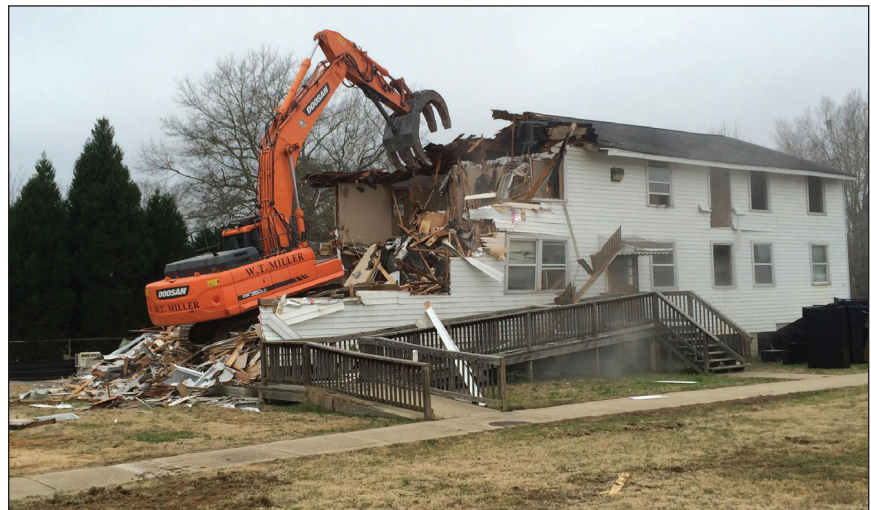
Soldiers Plaza building 2602, a World War II wood building used most recently as an administrative building, is demolished at Fort Moore, Georgia, under the Facilities Reduction Program.
