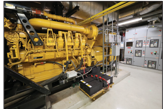
Pictured is a backup generator in a hospital mechanical room. The OMEE program maintains the facility and performs preventive maintenance repairs on these types of systems.
