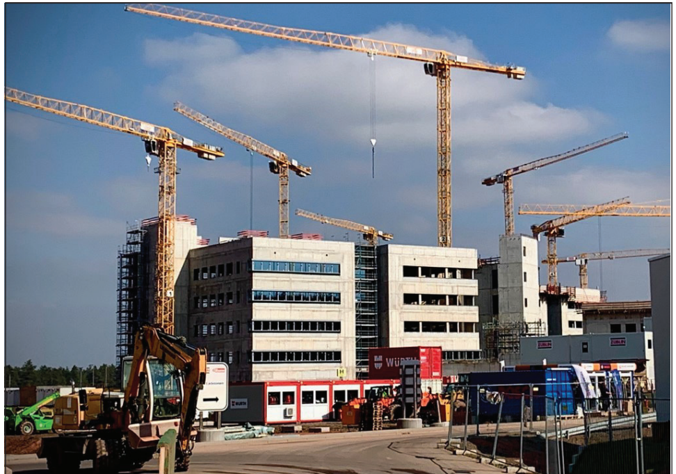
Outside the Outpatient Building Construction, Rhine Ordnance Barracks Replacement Medical Center, Ramstein, Germany.
