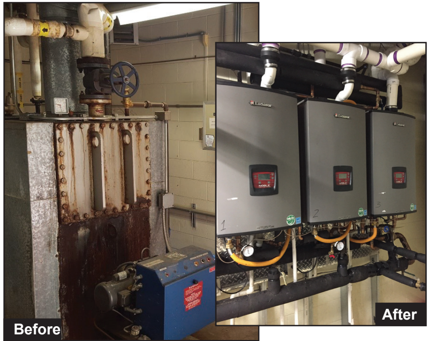
Replaced the 990,000 BTU input 70 percent efficient water heater (left) with 740,000 BTU input 90 percent efficient tank-less water heaters (right) to perform the same water heating requirement.
