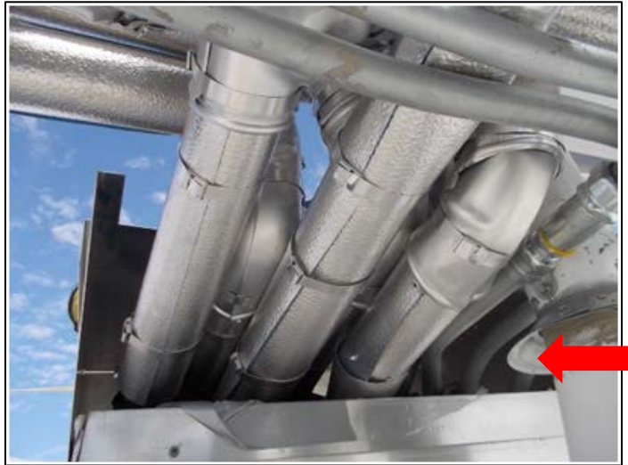
Counter flashing involved with arrow indicating location.
