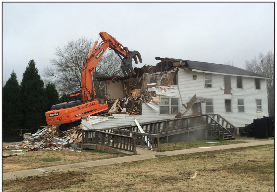
Soldiers Plaza, Bldg. 2602, a World War II wood building used most recently as an administrative facility, is demolished at Fort Benning, Georgia, under the Facilities Reduction Program.
